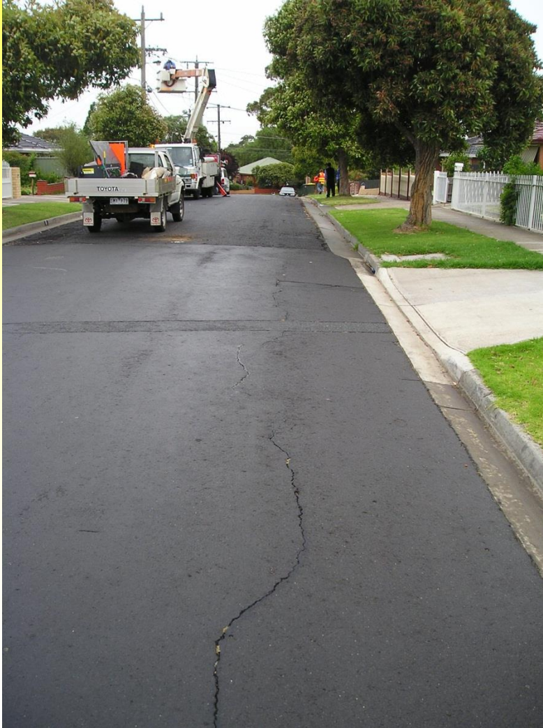
Longitudinal and Transverse cracking
